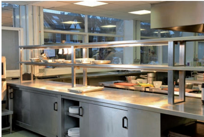
Figure 3.2 Example of a hotplate area
